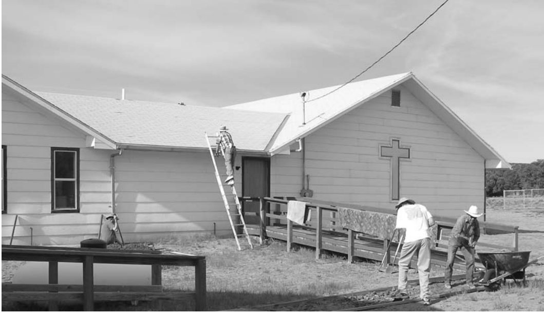
Working on a ramp and the roof at the church at Pinedale
